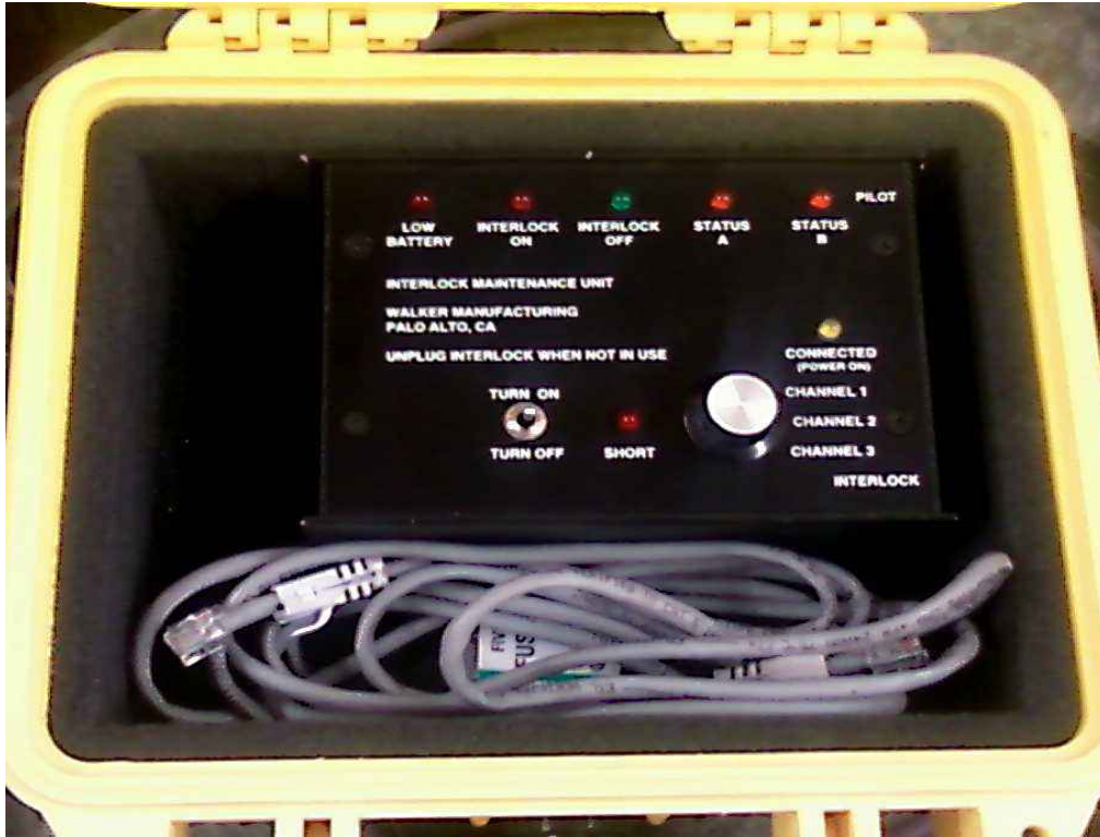
Figure 3 Walker Maintenance Unit (located in CA-2).
